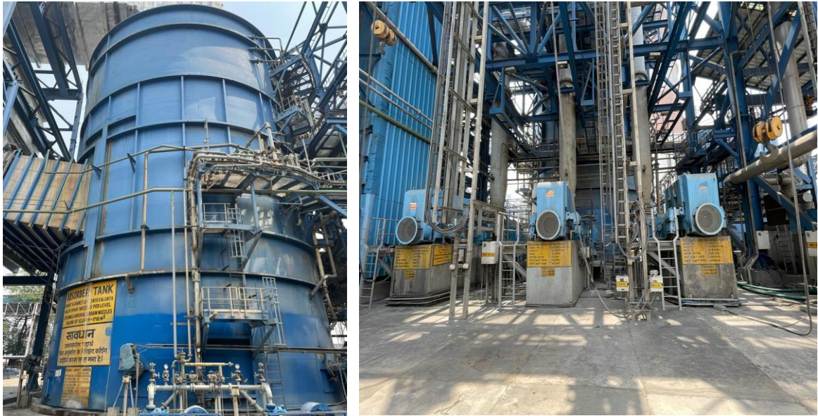
FIGURE 6: ABSORBER AND RECIRCULATION PUMPS
