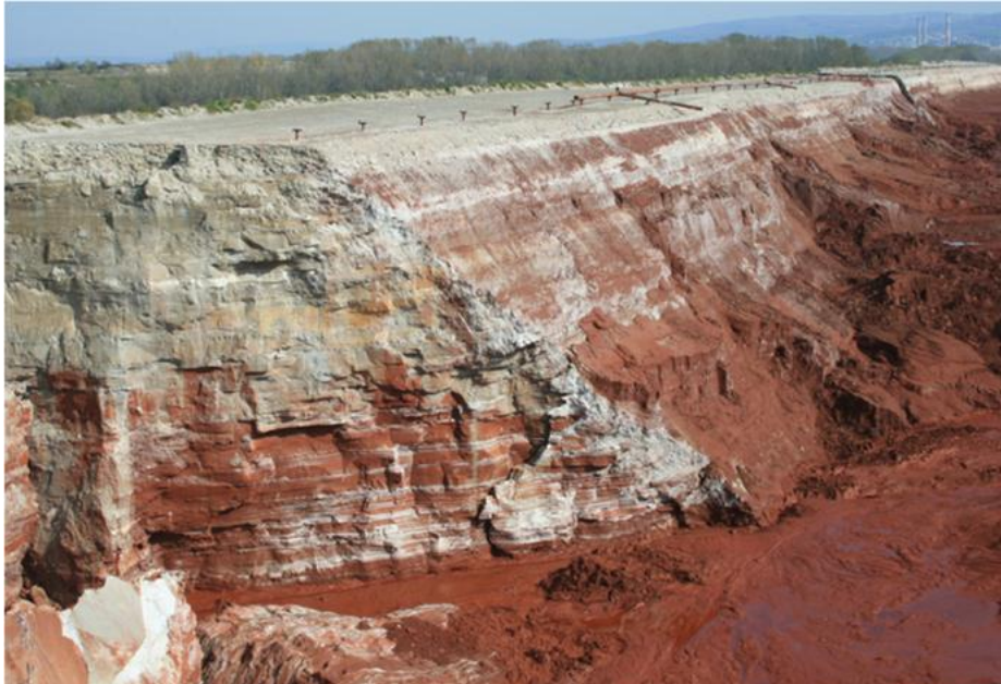
Figure 32: Material of the northern embankment of Reservoir No. 10 after the embankment failure
