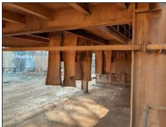
Hoppers for Red Mud dumping into Trucks
