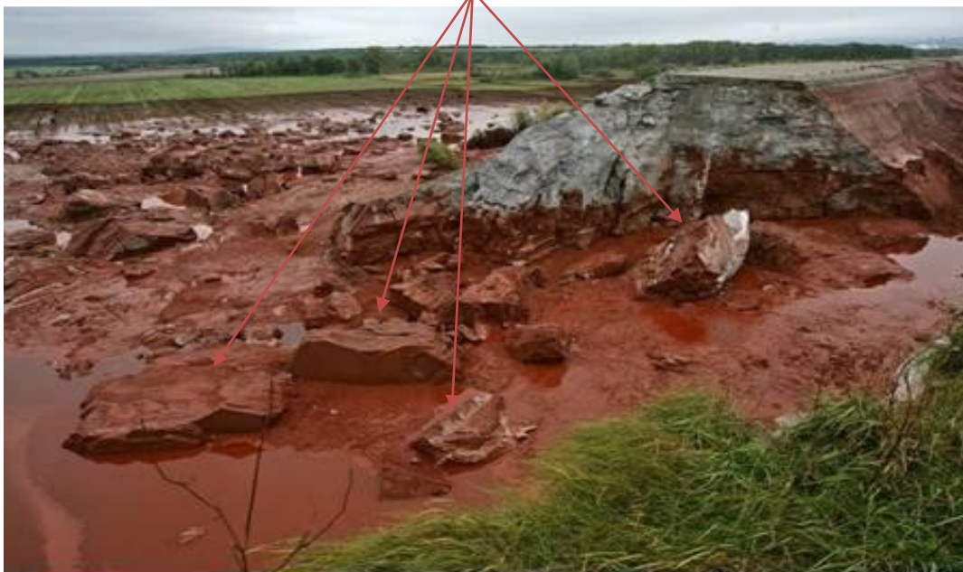
Figure 33: Material of the northern embankment of Reservoir No. 10 with fly ash after the embankment failure
