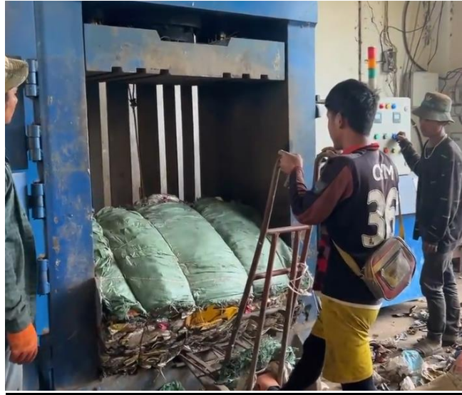
Pic: Baling machine at ULB
